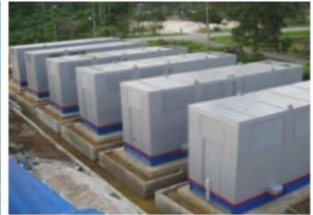
Containerised power generation (6MW)
